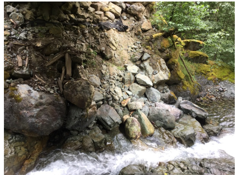
Downstream left bank riprap failure
