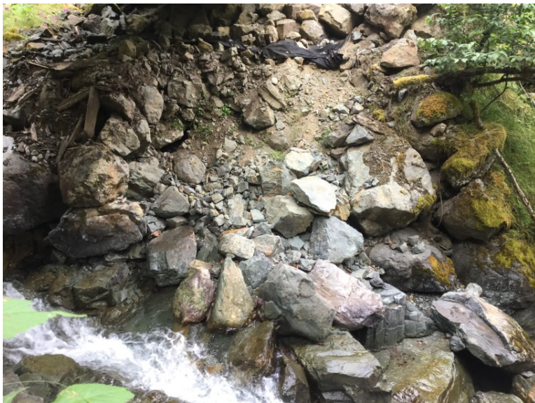
Downstream left bank riprap failure
